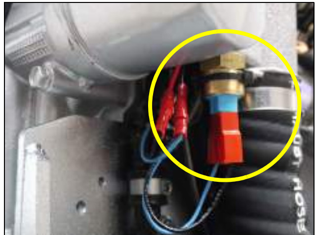
Fig. 4.3.4-2: Thermo-switch at exhaust connection
