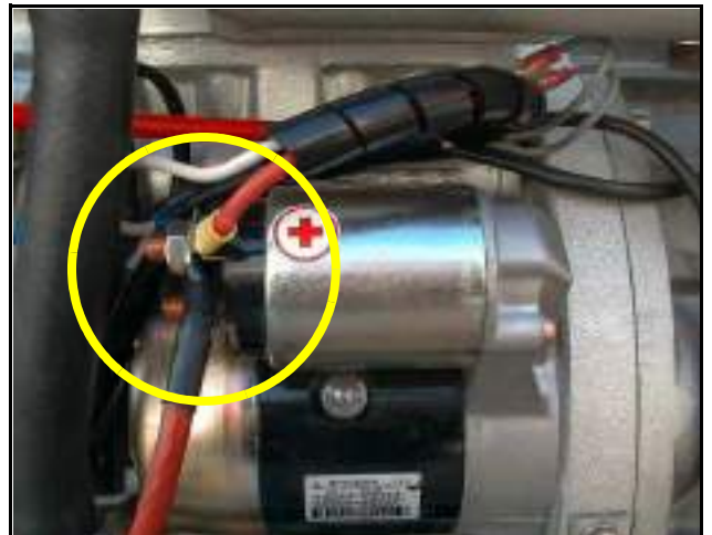
Fig. 6.10.1-1: Positive Battery Cable
