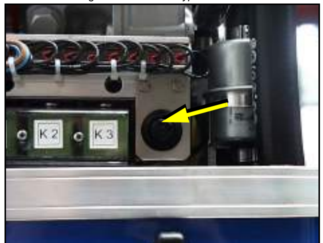
Fig. 8.9.2-1: Failure Bypass Switch
