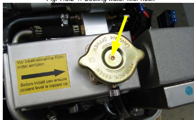
Fig. 7.5.2-1: Cooling water filler neck
