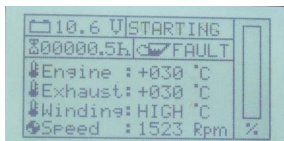
Fig. 17.1.1-2: Warning: „Winding temperature too high“
