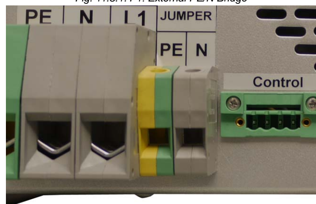
Fig. 11.5.1.4-1: External PE/N Bridge
