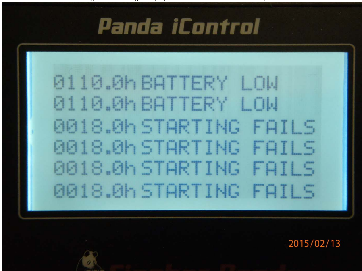
Fig. 14.3.7-1: Image: Display of the stored errors on the control panel
