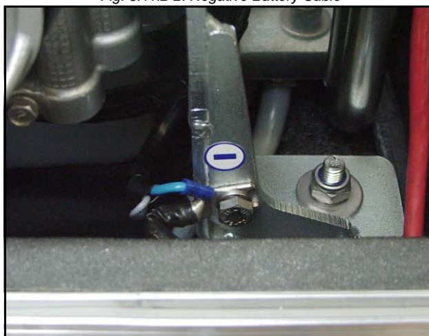
Fig. 5.11.2-2: Negative Battery Cable
