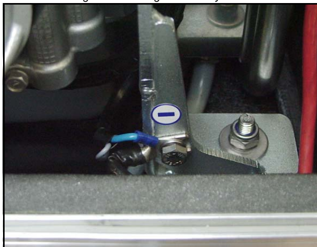
Fig. 5.11.1-2: Negative Battery Cable
