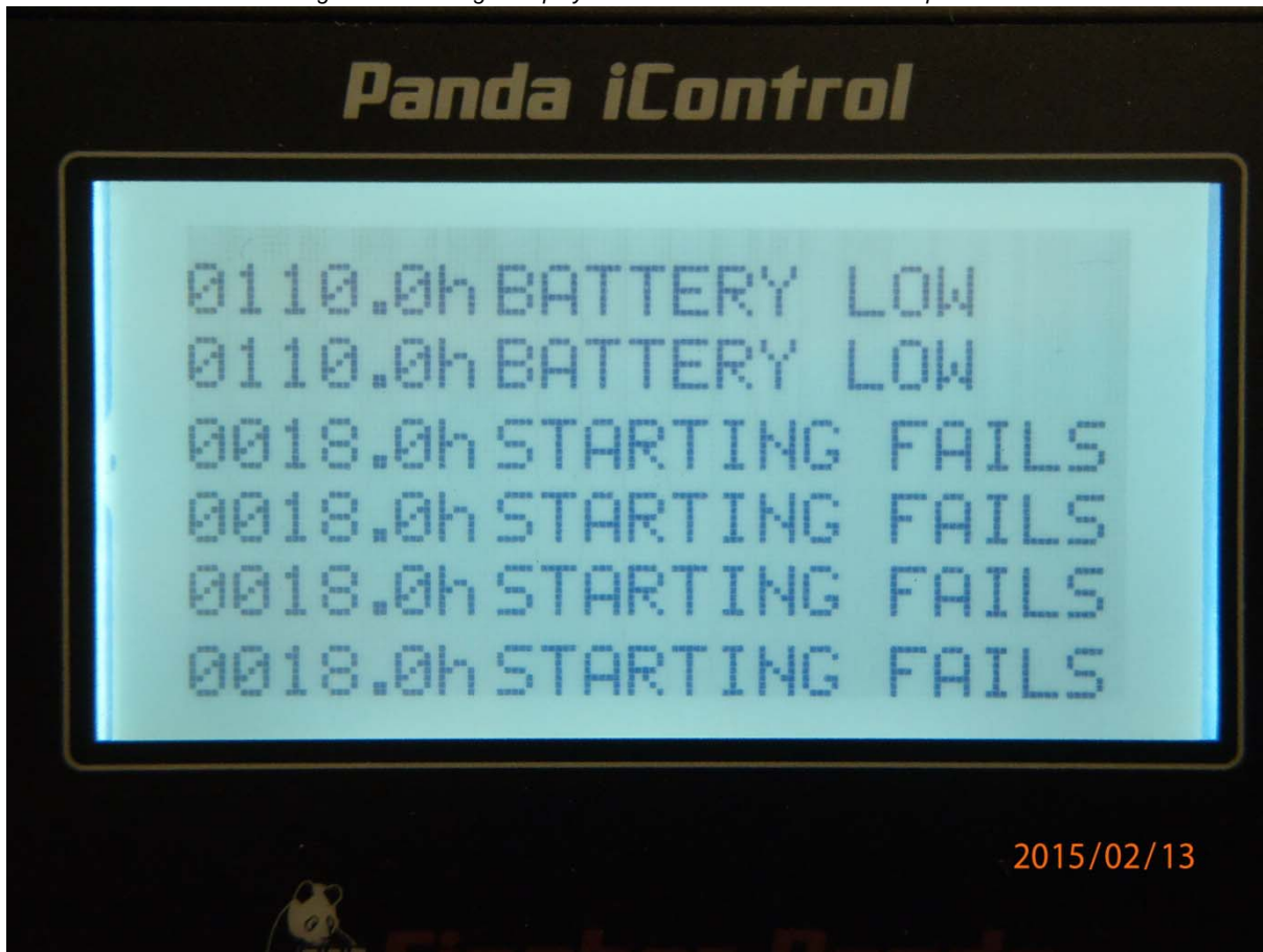
Fig. 15.3.7-1: Image: Display of the stored errors on the control panel
