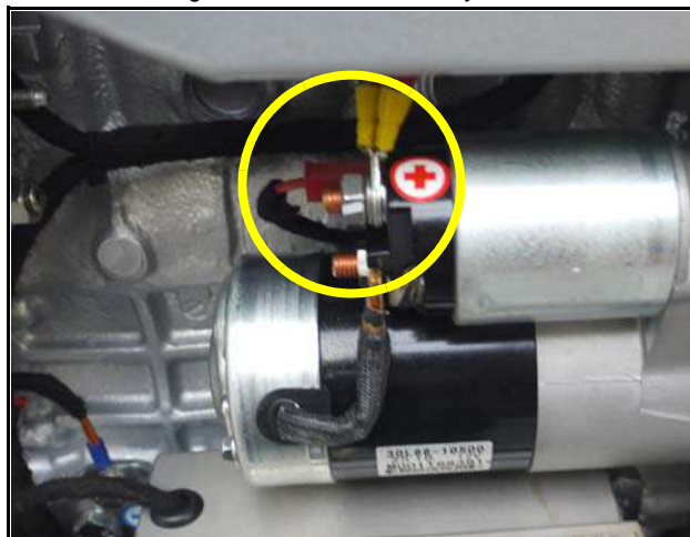
Fig. 6.14.1-1: Positive battery cable
