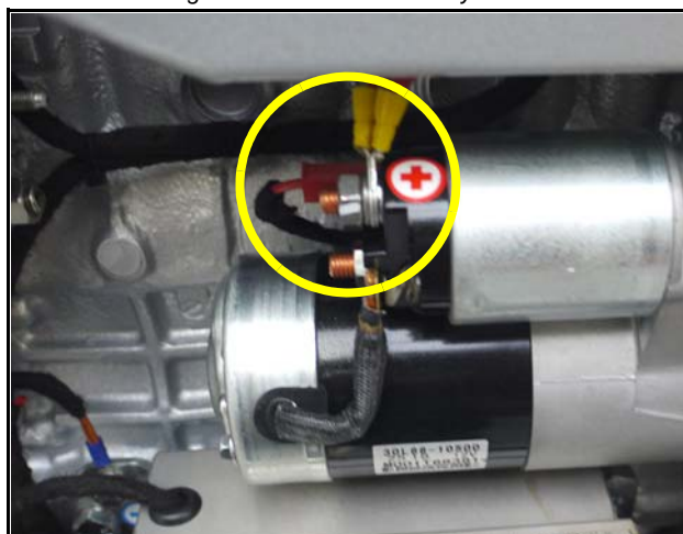
Fig. 6.14.1-1: Positive battery cable
