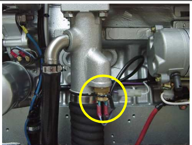
Fig. A.3.8-3: Thermo-switch at exhaust connection
