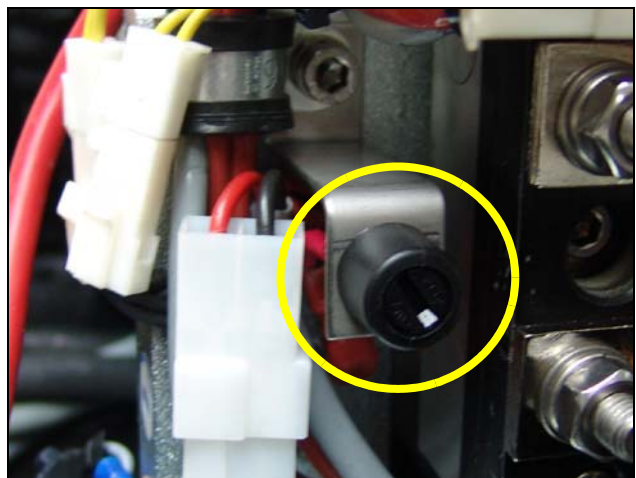
Fig. 5.3.6-11: Fuse for Measurement Voltage
