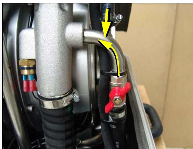
Fig. 5.3.2-8: Injetion Nozzles for Cooling Water
