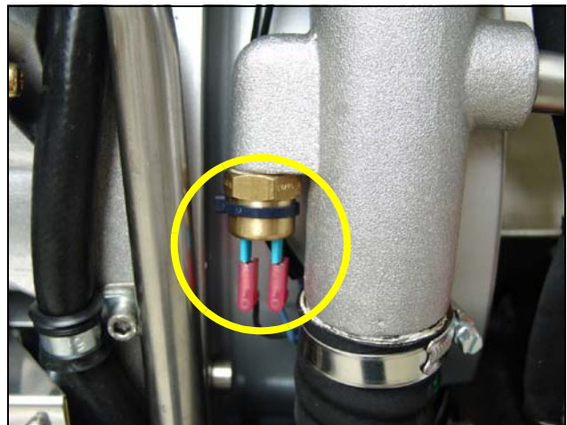
Fig. 5.3.7-3: Thermo-switch at Exhaust Connection
