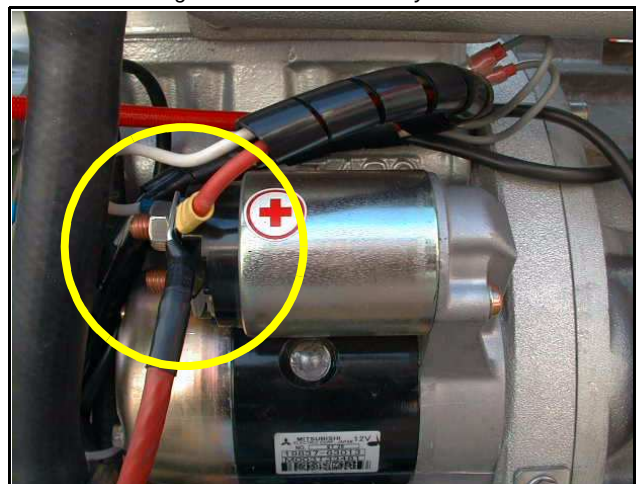
Fig. 5.8.2-1: Positive Battery Cable
