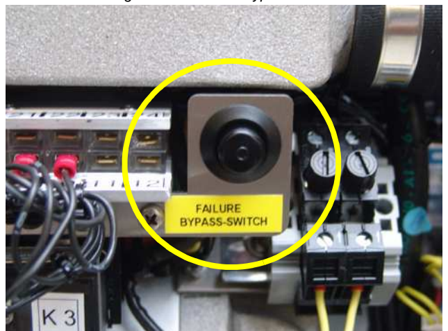
Fig. 4.2.5-9: Failure bypass switch
