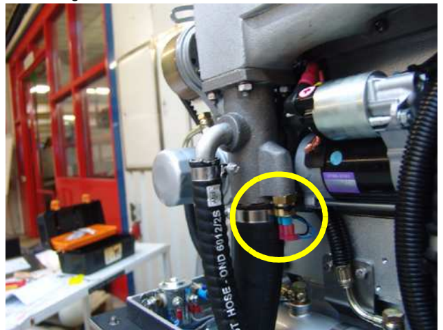
Fig. 4.2.5-3: Thermo-switch at exhaust connection
