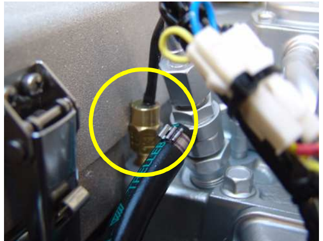
Fig. 4.2.5-1: Thermo-switch at cylinder head
