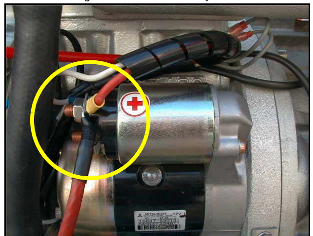
Fig. 6.10.1-1: Positive battery cable
