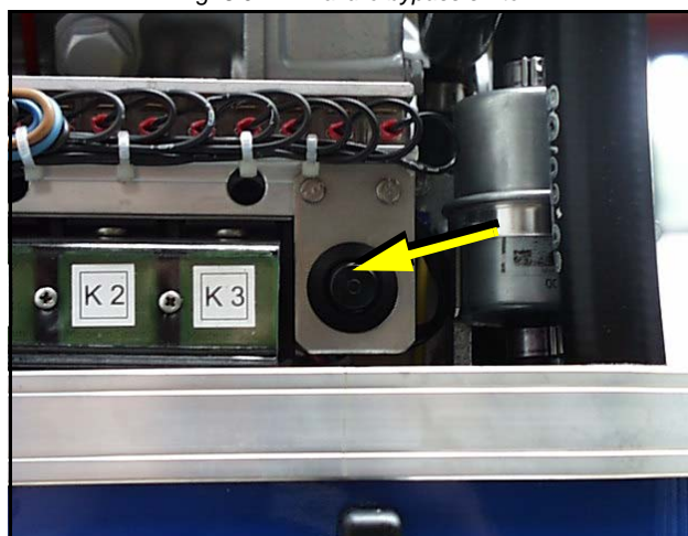
Fig. 8.9.2-1: Failure bypass switch
