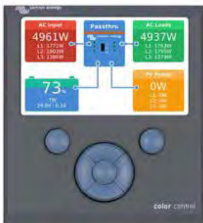
Color Control panel, showing a PV application
