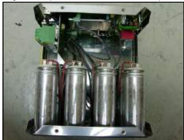
Fig. 7.11.3-2: Opened AC Control Box from Panda 30 upwards
