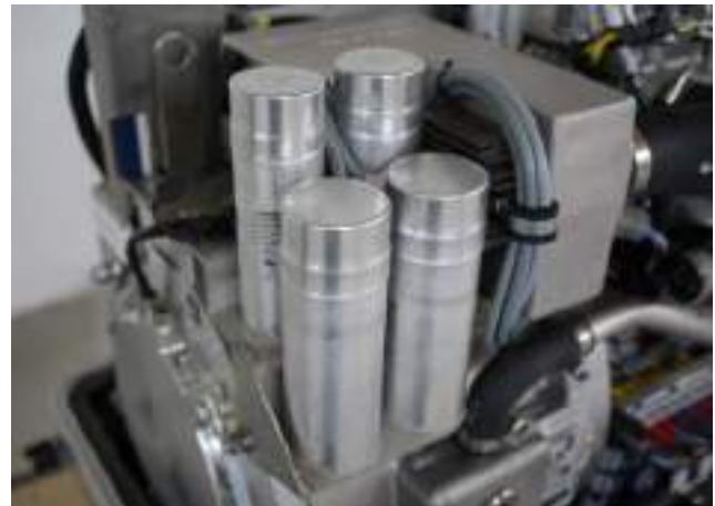
Fig. 7.11.4.1-2: Capacitors at the Panda 6000 ND PMS
