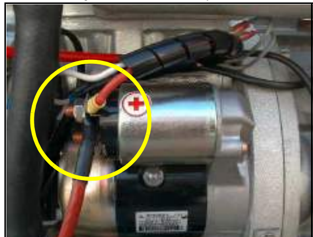
Fig. 7.10.1-1: Positive Battery Cable
