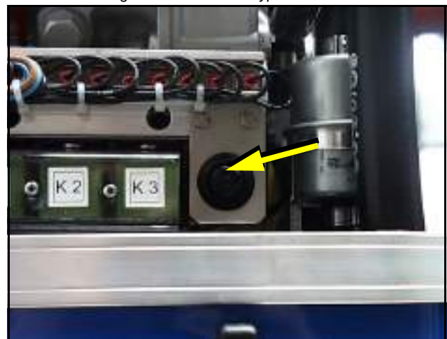
Fig. 10.9.2-1: Failure Bypass Switch
