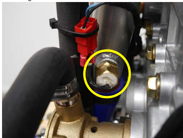
Fig. 4.3.6-2: Thermo switch at exhaust connection
