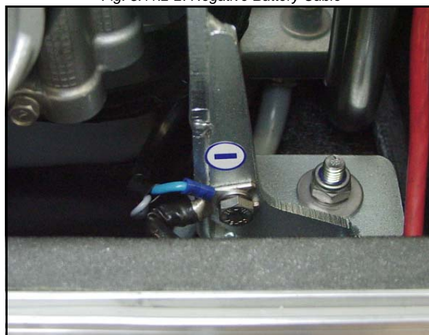
Fig. 5.11.2-2: Negative Battery Cable
