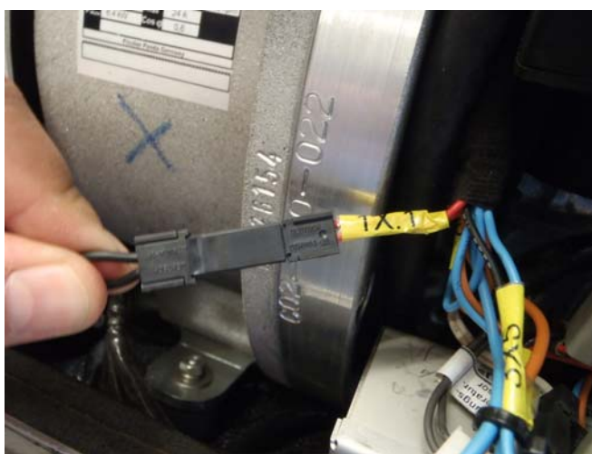
Fig. 13.5-1: Not Stop bridge in the cable harness
