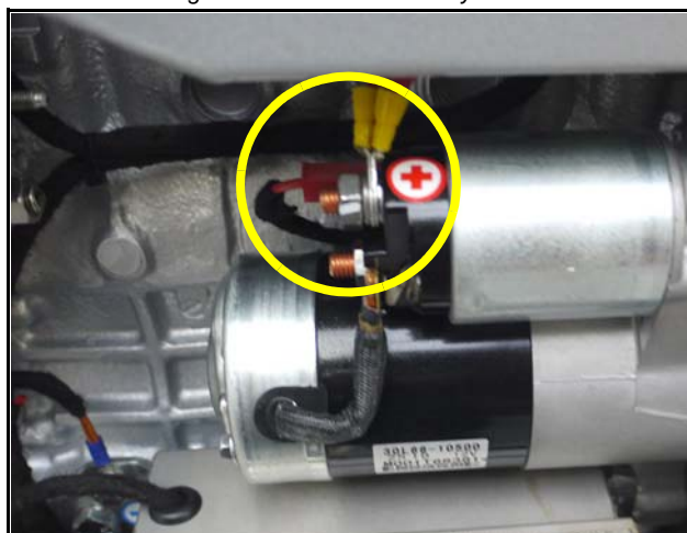
Fig. 7.13.1-1: Positive battery cable
