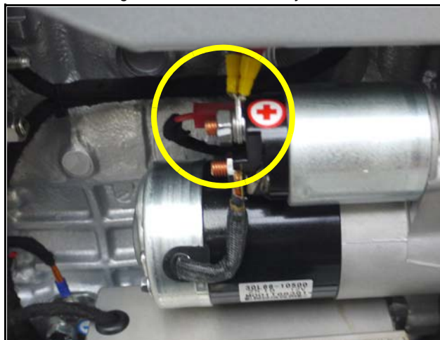
Fig. 6.13.1-1: Positive battery cable
