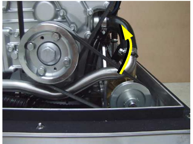
Fig. A.3.3-7: Internal cooling water pump
