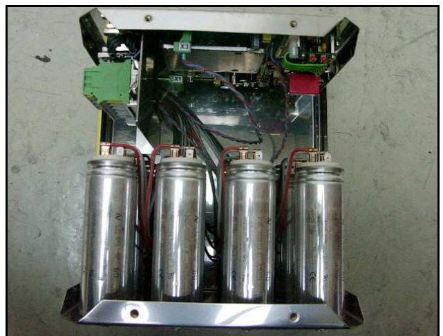
Fig. B.8.3-2: Opened AC Control Box from Panda 30 upwards
